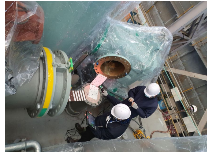
45° 곡관, 450/650A Cargo Pipe in P/RM
